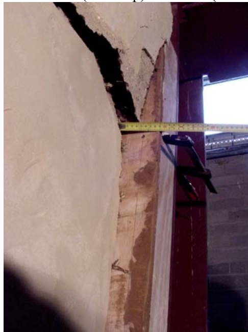
Figure 20: View of earth rendered wall (near top) after test (Source S. Overmeyer)
