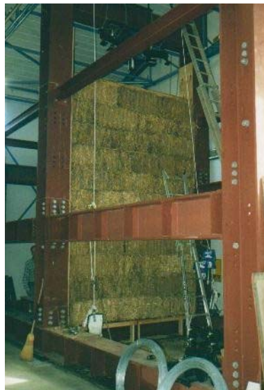
Figure 1 General view of steel test frame and partly completed wall for two-storey wall (Photograph: P. Florence)
